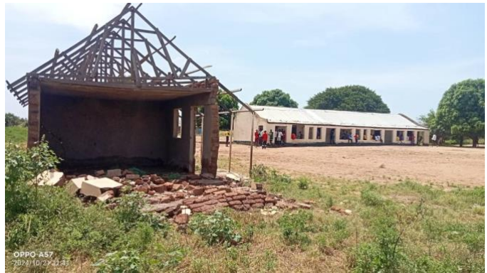
Damage from Flooding
